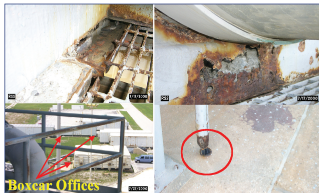
Figure 3.2.1. Launch Pad Corrosion and Boxcar Facilities.
